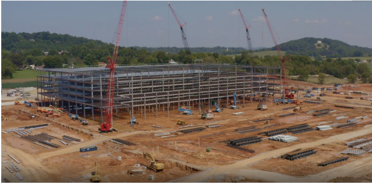
Pictured above shows the steel framing for approximately 25% of the footprint for Amazon distribution facility.
